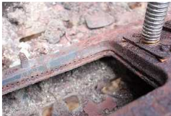
My Falcon burner could be brushed down and the gas ports reamed with drill bit. Then it should be blown out with compressed air. It isn't worth it to me.
