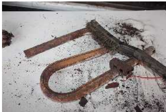
This is a Ducane burner with a portion brushed off. It needs a total brush down and to be blown out.
