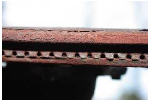
Members Mark burner showing rusted gas ports partially closed.
